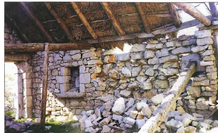
37 Ruševina stambene prizemnice s pokrovom od ražene slame Tumbledown residential ground floor building with roof of rye thatch
